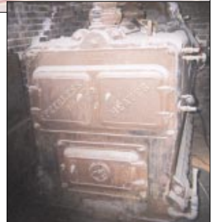
The original 1930s boiler of the historic Wilson Theatre.
