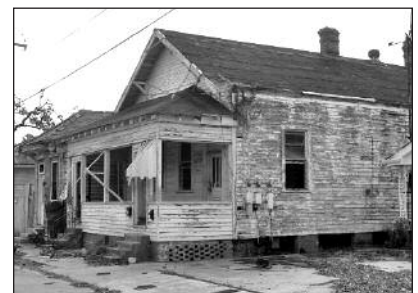
Just one of the thousands of homes that had been entirely covered with water.
